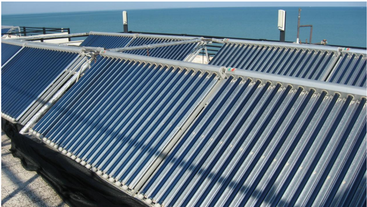
Fig. 2.1 Example of a solar thermal system with evacuated tube collectors installed in Italy
